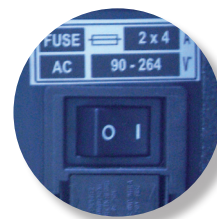
Main general switch
